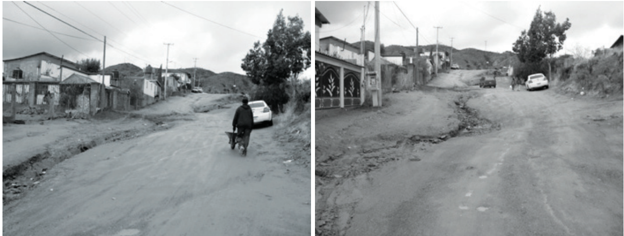
Figures 2-3a and 2-3b. Damage is evident on unpaved roads in a Nogales, Son., colonia after heavy rain (1/28/2010). Source: Photos by Jeremy Slack.
